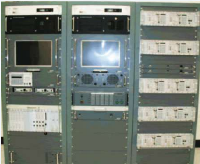
VHF Ground Radio Station
